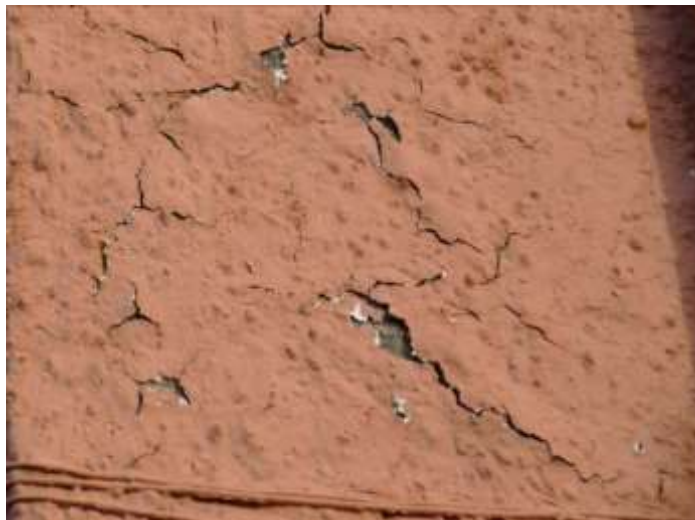
Cracked paint to roughcast render
