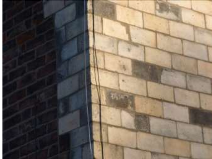
Damaged buff bricks to front elevation and hard cementitious pointing to gable
