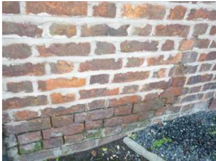
Hard cementitious pointing and eroded mortar
