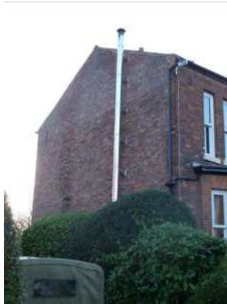
Unsuitable duct to gable wall of number 14
